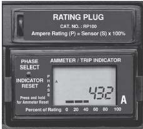
Combination Load Current Meter and Trip Indicator
