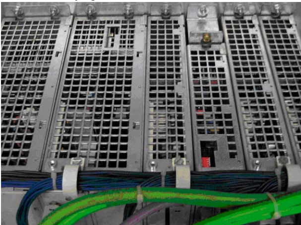
Good cable laying on SIMODRIVE
